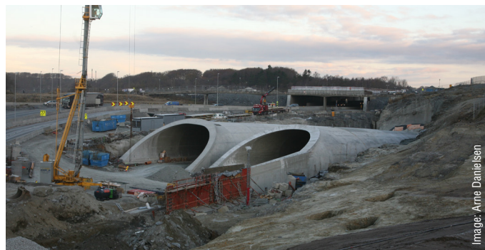
The Norwegian Public Roads Administration is building new tunnels in Stavanger and Bravida is providing all electrical installations in the Eiganes and Hundvåg Tunnels. Eiganes Tunnel will direct traffic outside Stavanger, while the Hundvåg Tunnel will be an undersea tunnel linked to the mainland. Bravida's work in Stavanger will include fitting 364,000 metres of cabling and installing 4,000 electrical fittings, 840 LED lights, 450 information displays and 240 surveillance cameras.
