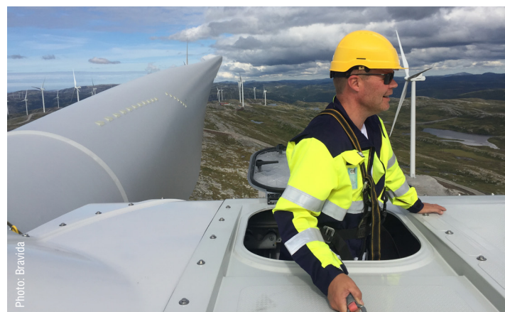
Europe's largest land-based wind farm is being constructed in Central Norway. Once fully operational, the facility will supply 170,000 households with electricity. Bravida has been contracted to supply seven electrical substations that will collect 33 kV from the wind turbines and transform up to 132kV for the central grid. The facility is due to enter service in 2020.
