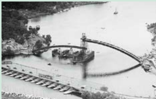
We are involved in the construction of the Traneberg Bridge, work on which starts this year.
