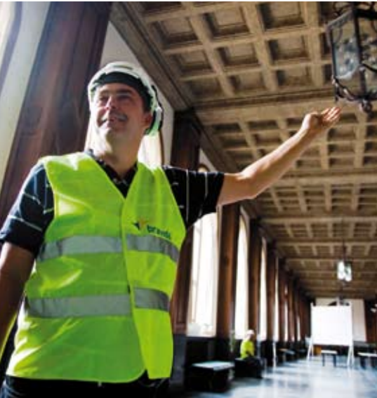
In the old post office building in Gothenburg, which is being converted into a state-of-the-art modern hotel, Bravida has overall responsibility for electrical installations, heating & plumbing, HVAC and sprinkler systems.
